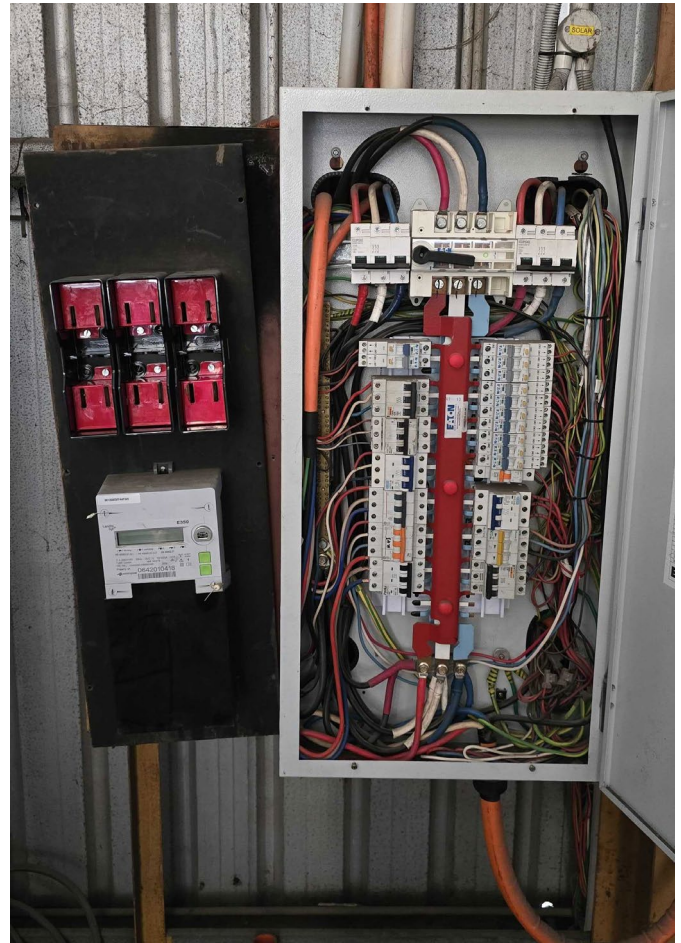
Figure 1. The electrical switchboard
