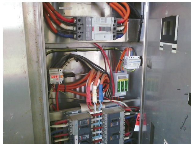
Figure 2. Surge diverter with high heat on device indicating leakage.
