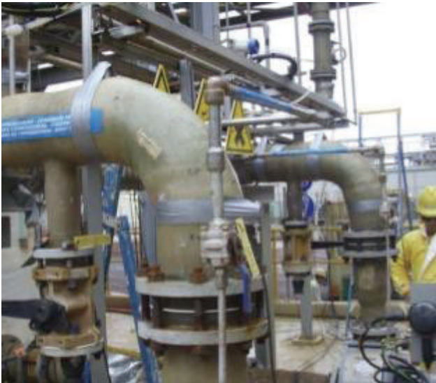
Figure 1 Identifying creep and fatigue cracking in high pressure pipelines.
