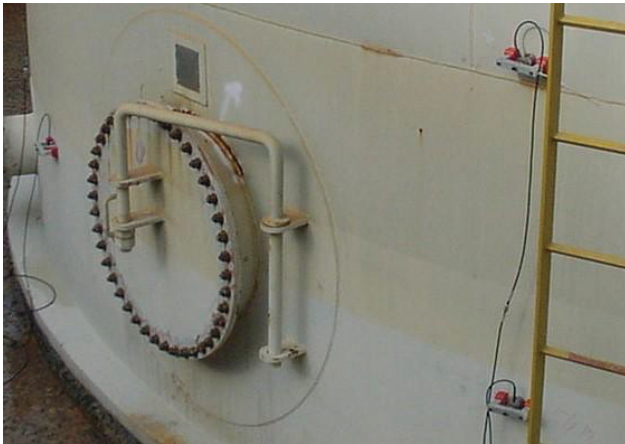
Figure 4 Storage Tank showing typical location of primary (lower) and guard (upper) sensor.
