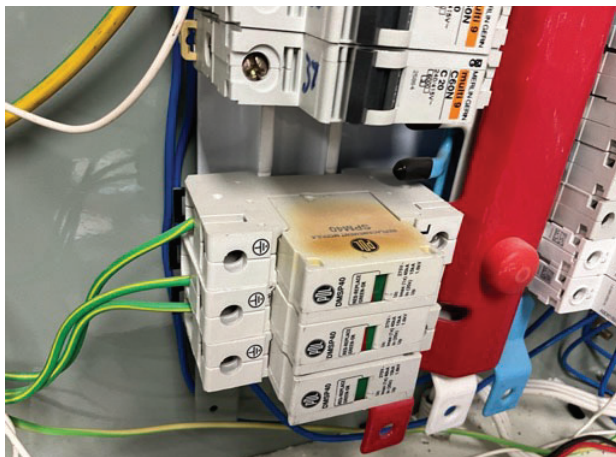
Figure 4. Surge diverter Thermogram and burn marks.
