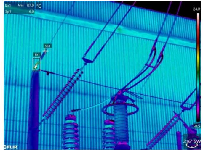
The earth wire connection to the top of an ground insulator at a 220KV Underground cable at a Power station is hot. Some current must be flowing in the earth at this point and there is some resistance associated with this termination.
